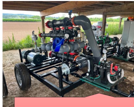
Trailer-mounted Pump, filter, and fertilizer injection
