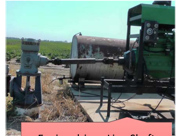
Engine driven Line Shaft Turbine
