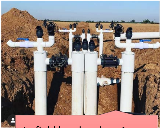
In-field headworks – 4 zone control valves & reliefs
